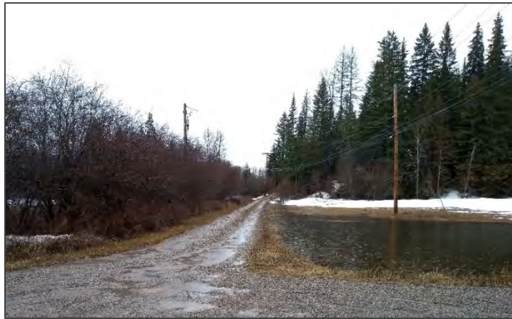
Figure 20. Spring Stormwater Collecting in a Field on the Proposed Trail Alignment, between Mt Fernie Park Rd and Lizard Creek.
